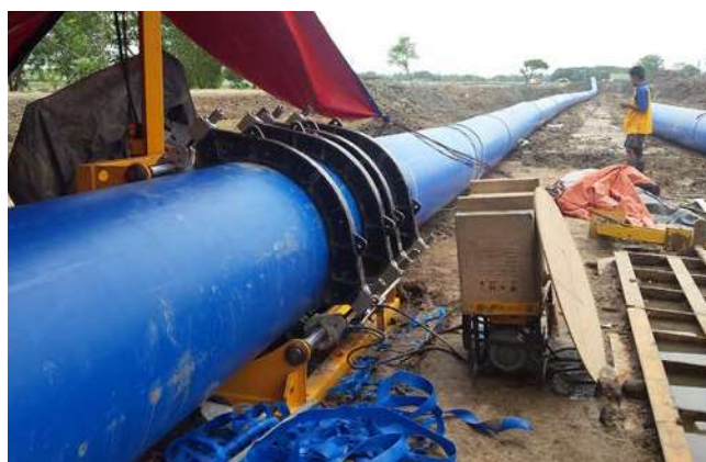
Multilayer 1,200mm OD PE100 with HSCR outer layer pipes being welded in Myanmar.
